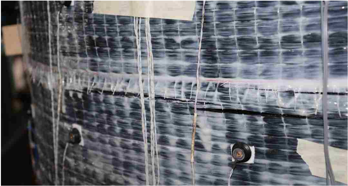
Figure 7-12. Close up view of split at 24-inches above cap beam
