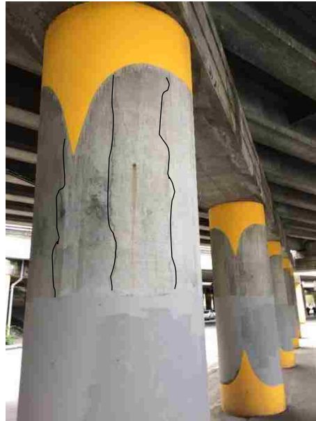
Figure 1-2. Longitudinal cracks on columns of Ravenna Bridge
