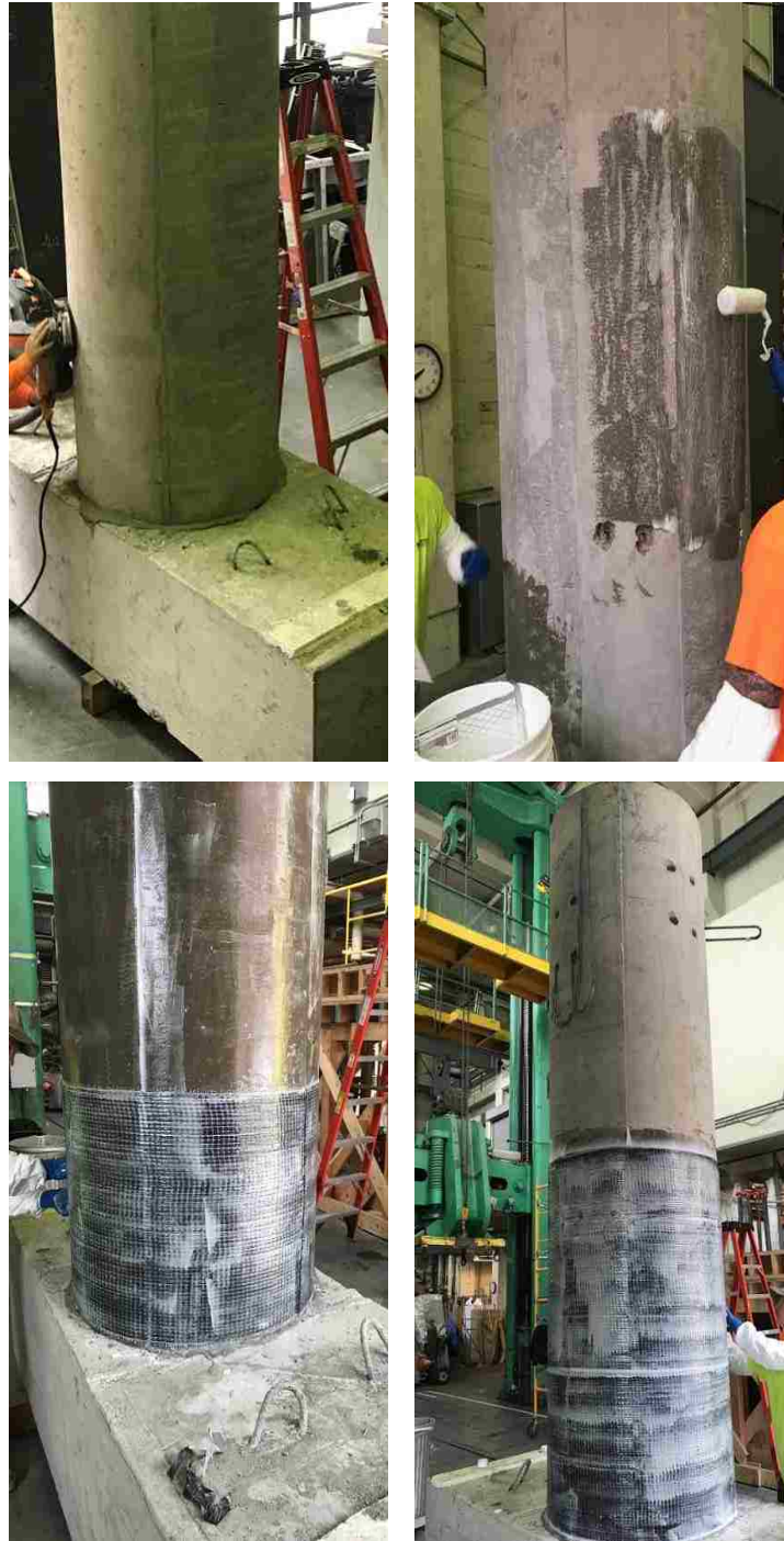
Figure 6-17. CFRP application: sanding concrete (top left), base epoxy (top right), first layer of CFRP (bottom left), finished epoxy (bottom right)
